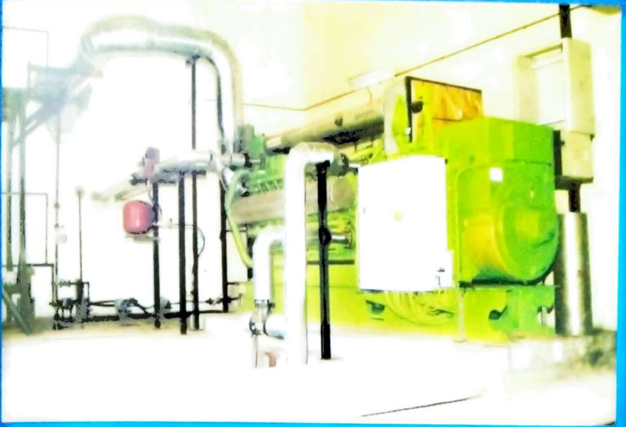
METHANE GAS ENGINE FOR PRODUCING ELECTRICITY - PERUNGUDI
